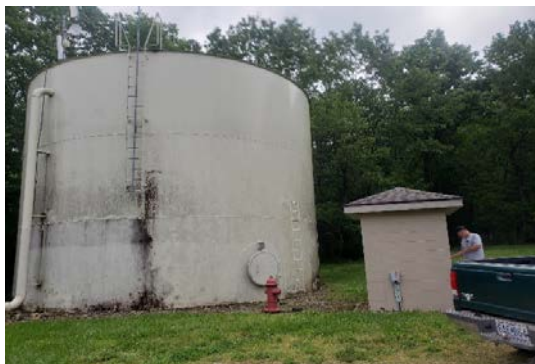
Water Storage Tank & Control Bldg
