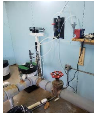
Well No. 1 Chem Feed
