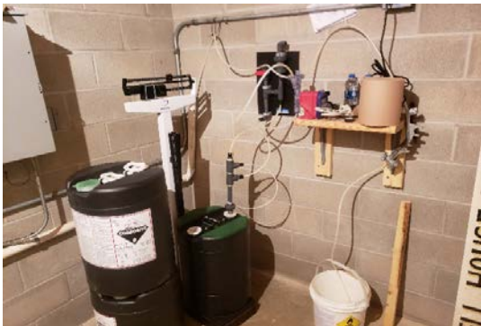
Well No. 2 Chemical Feed
